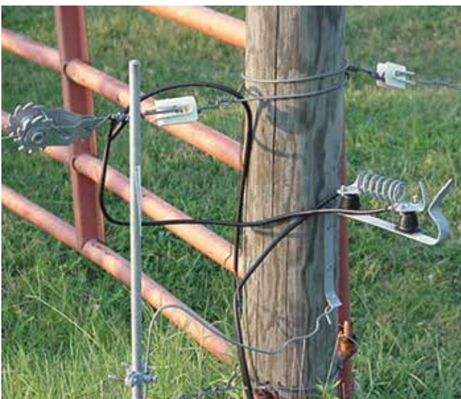
Figure 11-14. MWLA lightning protection.
