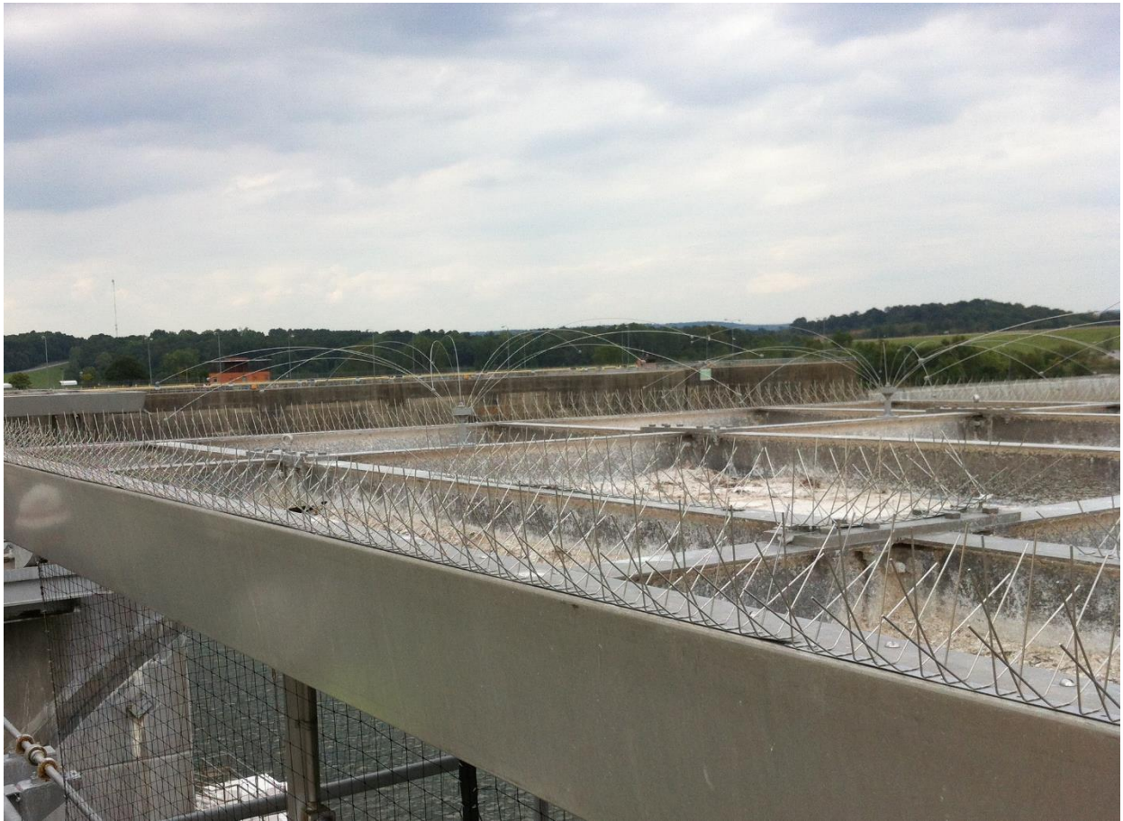
Installed bird spikes, netting, and wire deterrents on a lock and dam in Oklahoma (Photo courtesy of Stacy Dunkin, USACE).
