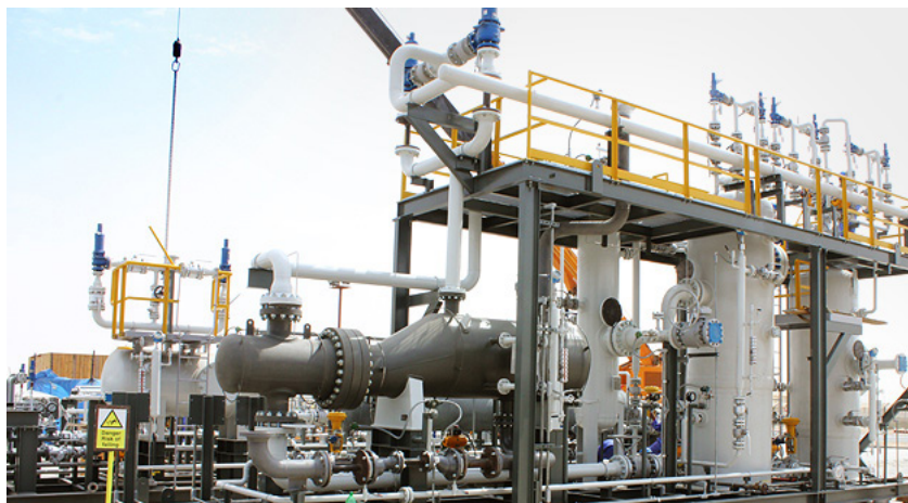
Figure 1-13: Natural gas sweetening unit
