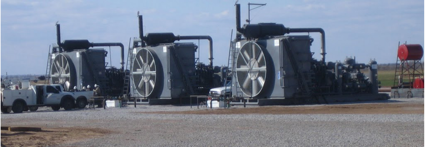
Figure 1-14: Natural gas compressors
