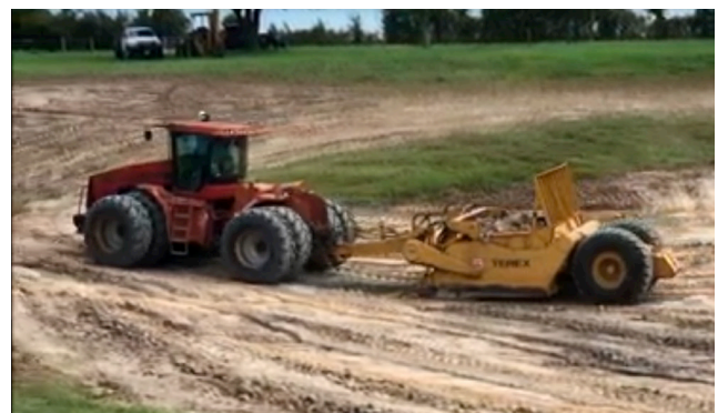
Figure 2. Pond contractors often remove soil from the basin area by scraper, which then is used to lay in 6-inch thick "lifts" to construct the embankment (dam). With proper moisture content and a sheepsfoot roller or dozer tracks, adequate compaction is achieved. An all-wheel drive tractor is an efficient equipment option often used by earthwork contractors doing pond work.
