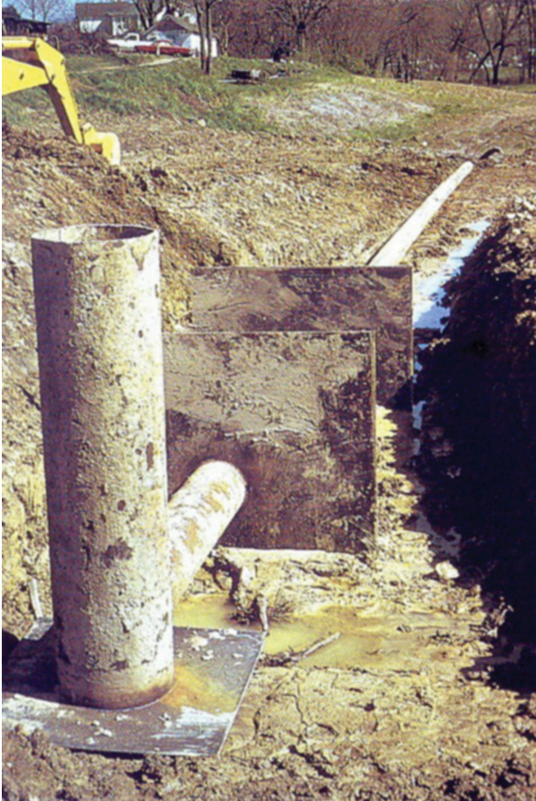
Figure 6. A smooth steel drain being installed in the early stages of dam construction. Proper drain installation involves proper slope, anti-seep collars (two shown here) and thorough compaction of each soil layer using a “jumping jack.” Beware of corrugated steel pipe: it is often short-lived due to corrosion. PVC or smooth steel pipe offers longer life. Avoid steel pipe that has been used for salt water. Image courtesy USDA - NRCS.
