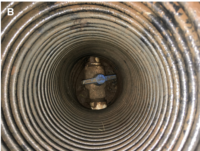
Figures 6a and 6b: The isolation valve is typically located in a small green valve box near the water meter or backflow preventer. This valve is in the closed position. Photos courtesy of Kevin Moore.
