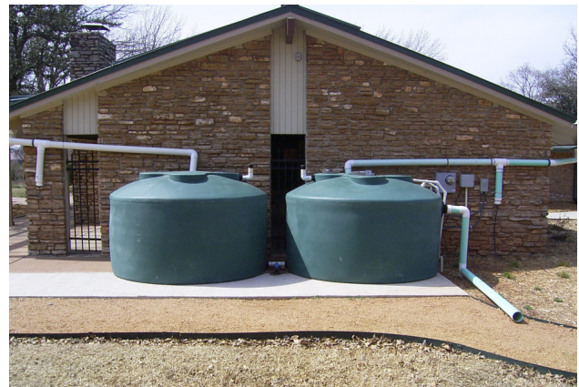
Figure 5: Rainwater harvesting system capable of capturing 2,200 gallons at the Xeriscape Gardens in Edmond, Oklahoma.
