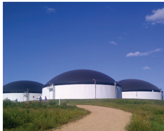
Figure 3. Three Complete Mix Reactors making up the Dane County Community Digester near Madison, Wisconsin.
