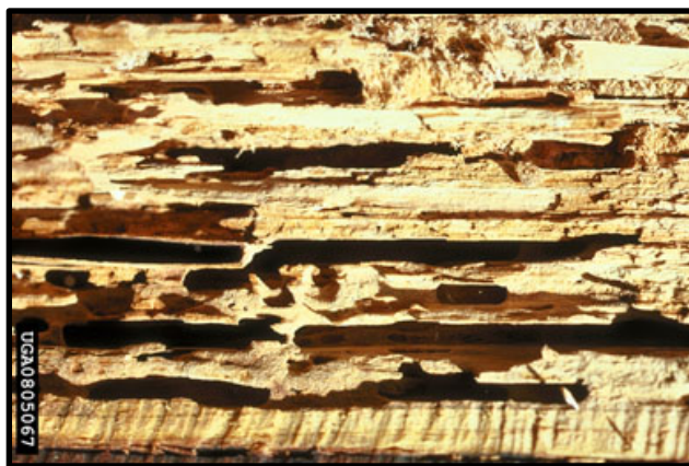
Figure 5. Carpenter ant galleries in building timber or log. Smooth-sided parallel galleries. [Photo courtesy R. Werner, Bugwood.org]
